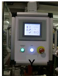
TOUCH SCREEN CONTROL PANEL
